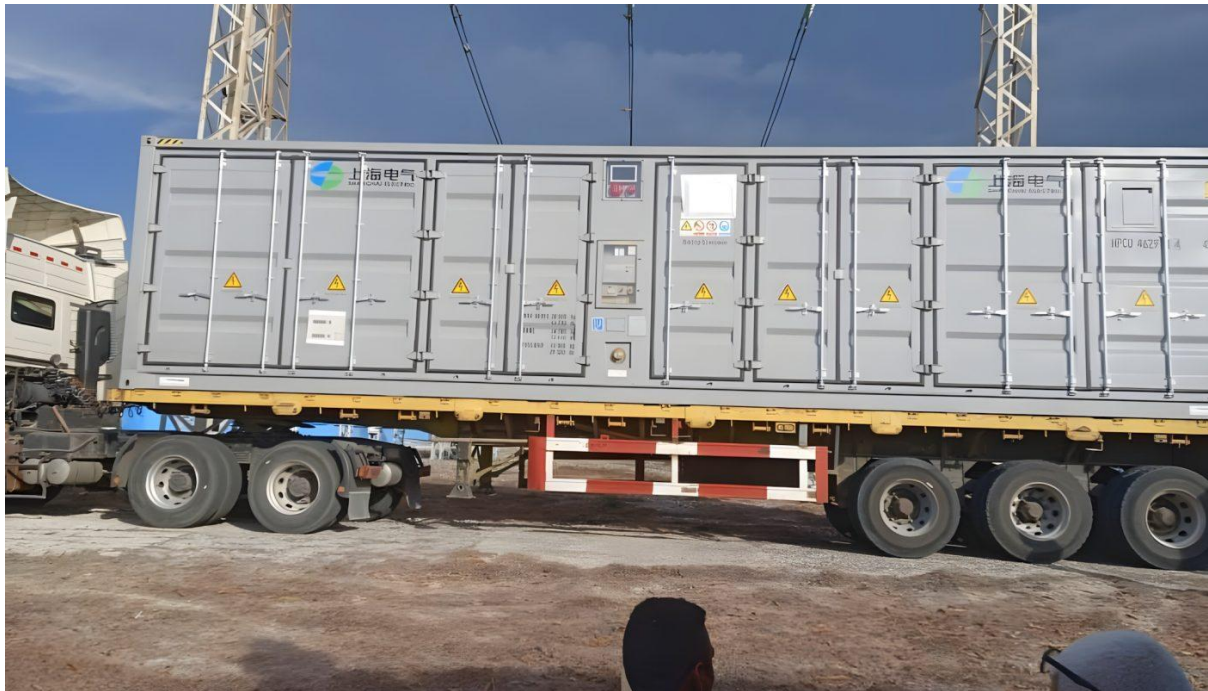
Part of the first battery storage systems (source: J.M. Solís/KI-scaled )
